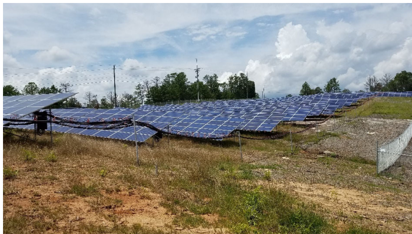
Example of a fixed tilt installation in Conyers, GA on solid rock with ground screw foundations
